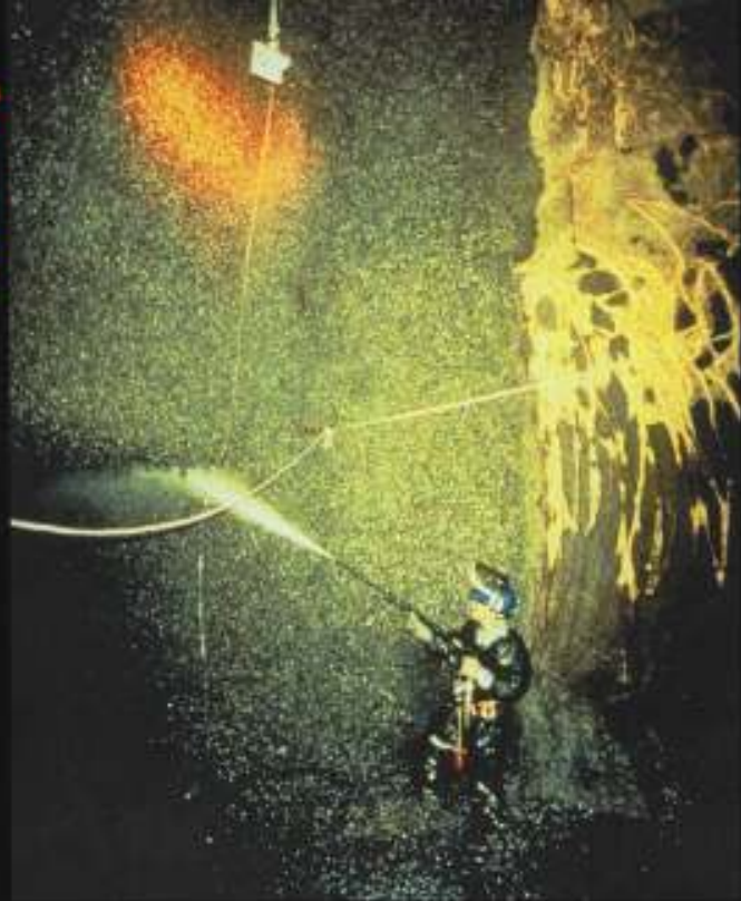
Eurasian zebra mussels, a leading cause of industrial damage in Canada and the U.S., blanket the walls of this water treatment plant.
